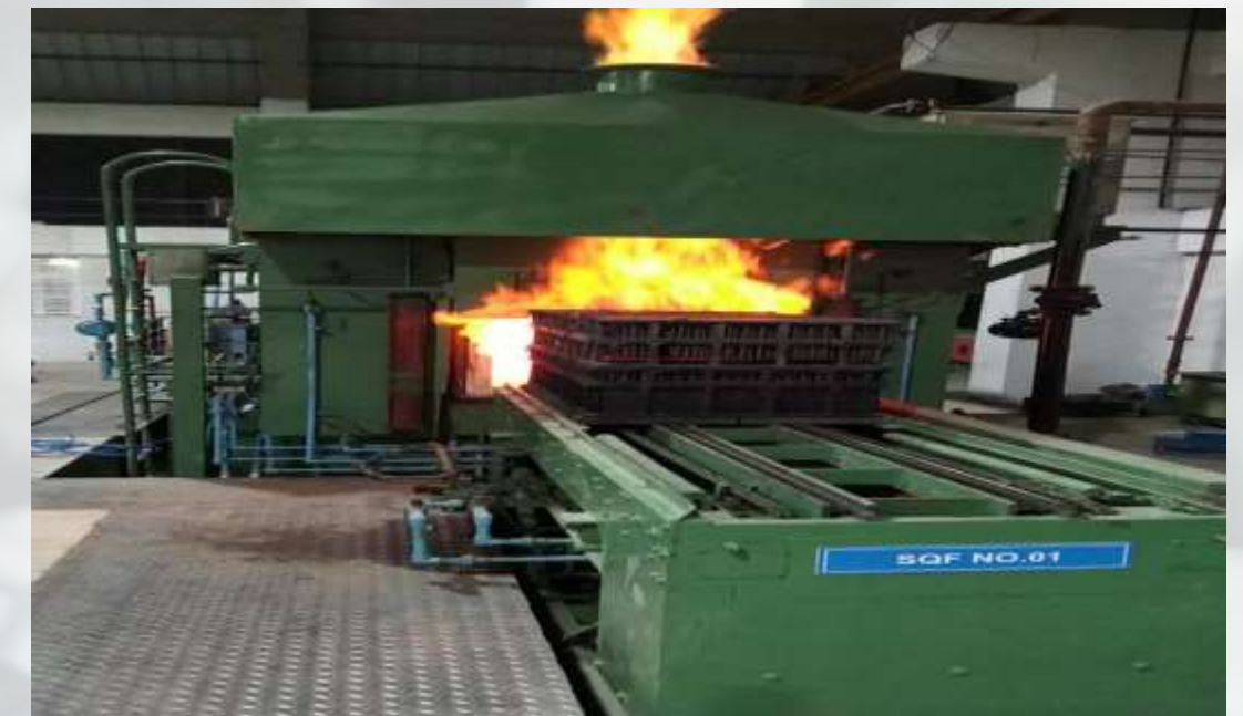
SEALED QUENCH FURNACE
